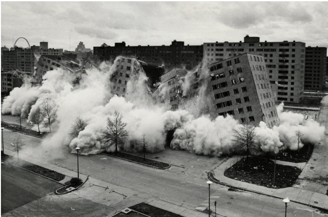
Implosion of first Pruitt-Igoe building, 1972. Courtesy of the St. Louis Post Dispatch.
